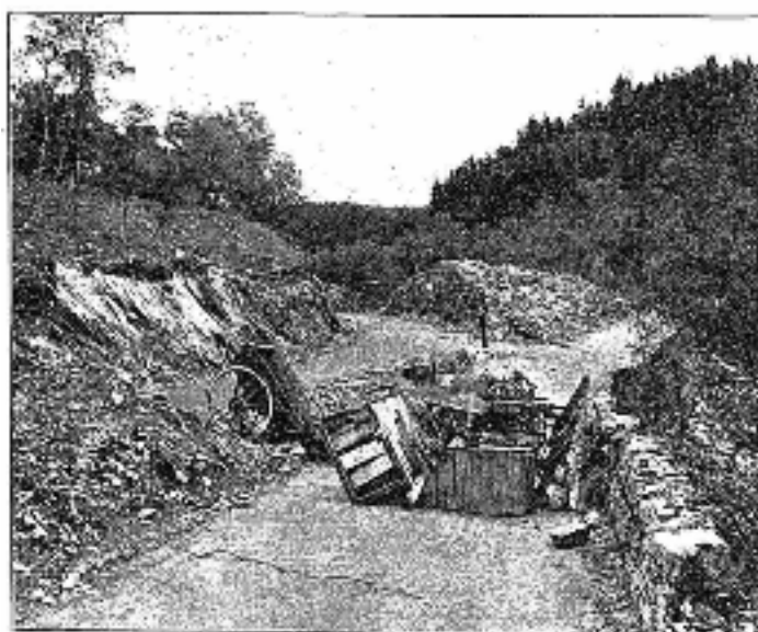
INVERNESS-CHIEF ROAD IMPROVEMENT. —Extensive reconstruction is being carried out on this narrow Ballachulish-Spean Bridge road. A section is now open to traffic, vehicles using the new road rolling on left.
